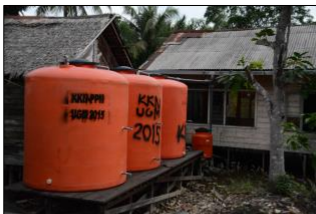
A configuration of tanks to service several families
